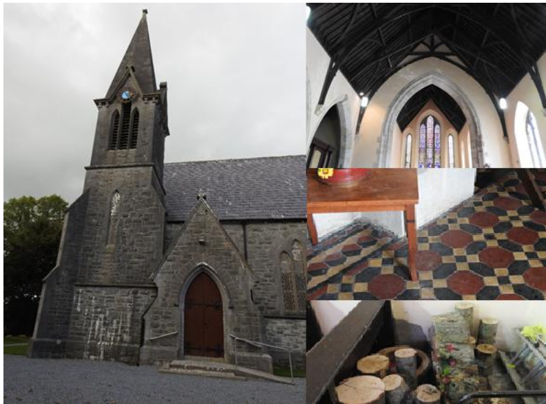
Figure 5.4 Lissadell Church, interior and examples of areas with urine stains and fouling by bats
