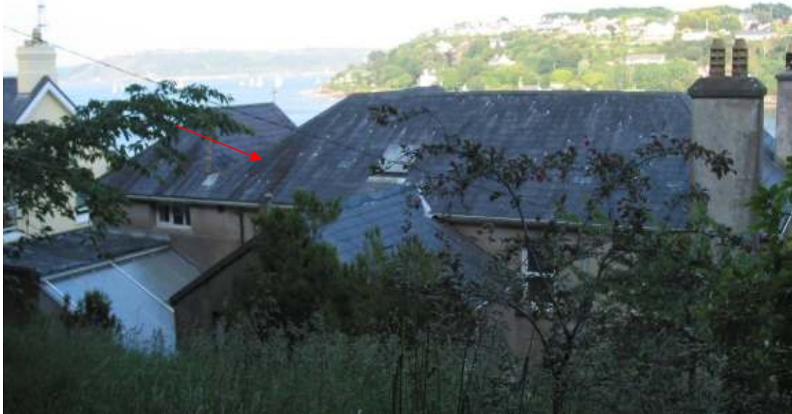
Plate 9: View of roof of Roost E (BCIreland Site Code 2005) with red arrow depicting possible location of exit point.
