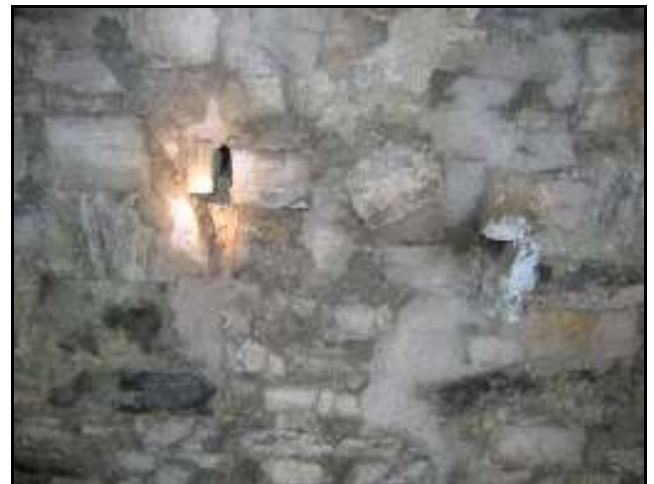
Plate 4: Repaired fissure under an arch of Lisconny Bridge – note how the stonework has not been covered by grout (Far Left)
